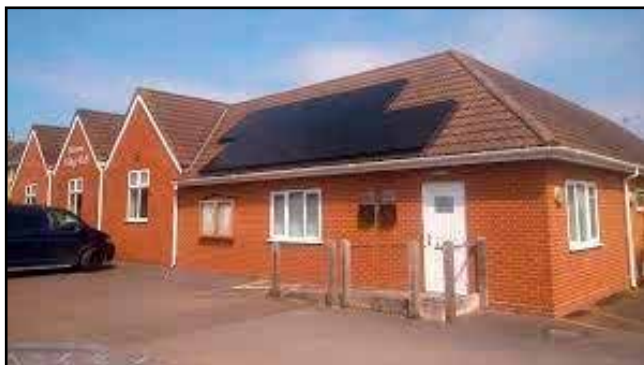
Solar panels fitted to Berrow Village Hall in Somerset
